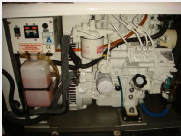
40' Cape Dory Generator
