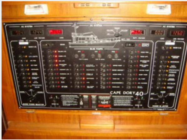
40' Cape Dory Electrical Panel
