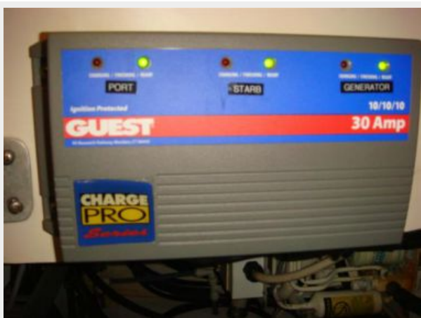
40' Cape Dory Battery Charger
