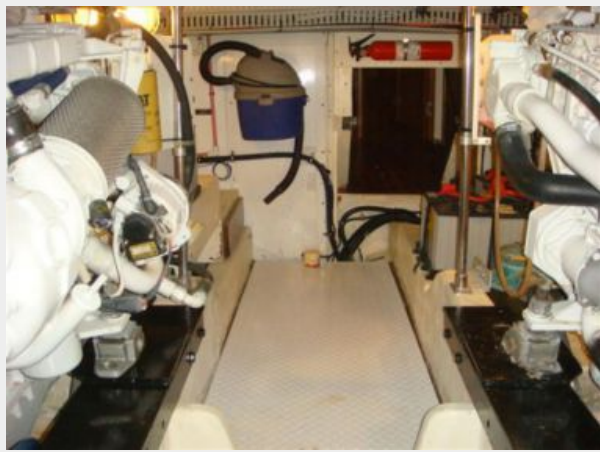
40' Cape Dory Engine Room Forward
