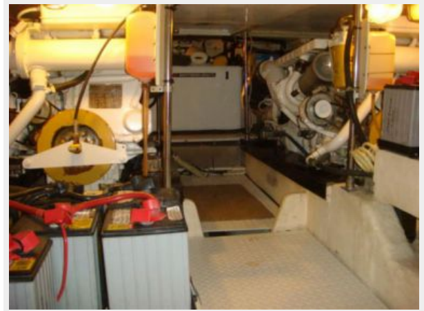
40' Cape Dory Engine Room Aft
