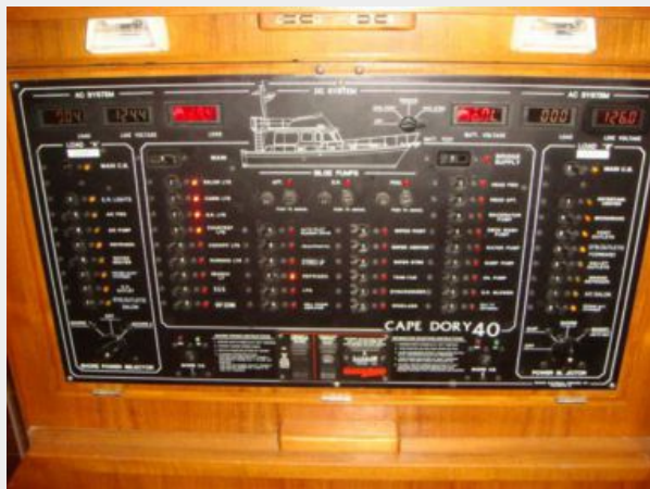
40' Cape Dory Electrical Panel
