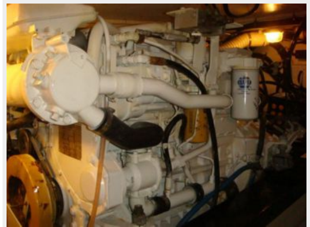
40' Cape Dory Starboard Main Engine
