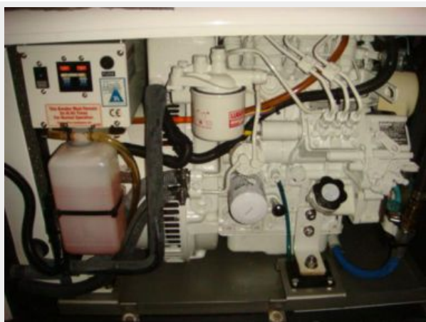
40' Cape Dory Generator
