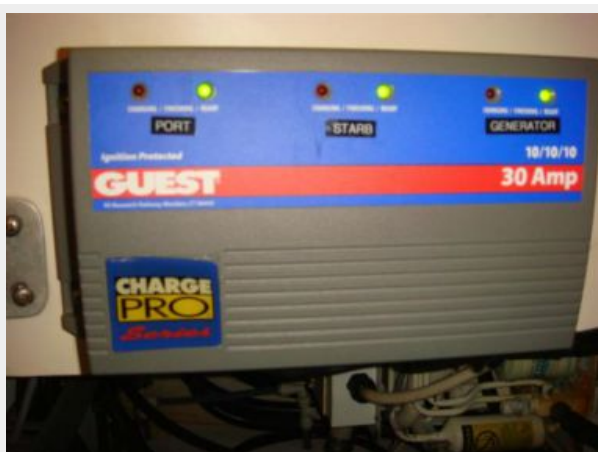
40' Cape Dory Battery Charger
