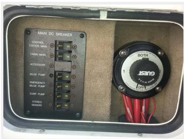
Cockpit control panel
