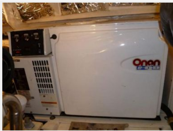
Onan generator w/ sound shield
