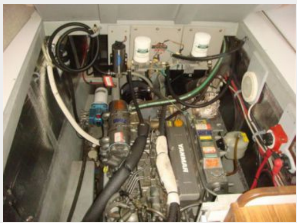
44' Endeavor Starboard Engine Compartment
