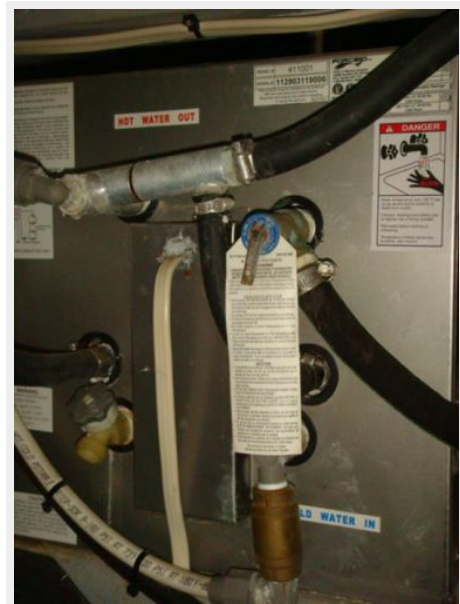
44' Endeavor Water Heater
