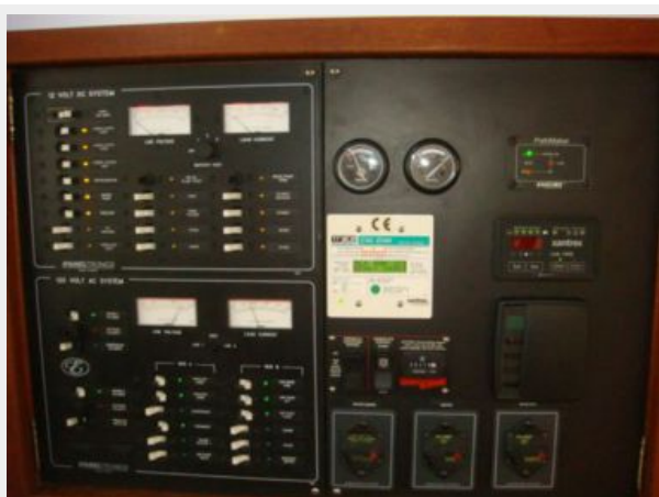
44' Endeavor Electrical Panel
