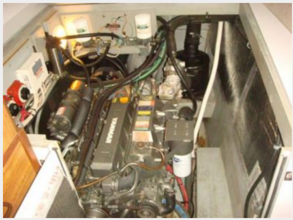
44' Endeavor Port Engine Compartment
