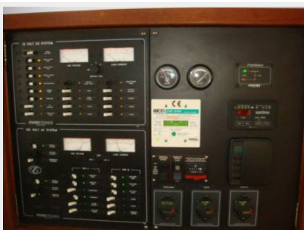
44' Endeavor Electrical Panel
