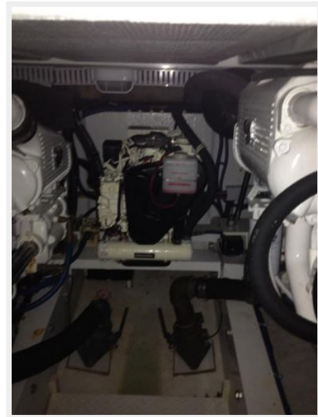
Engine & Mechanical Equipment 1
