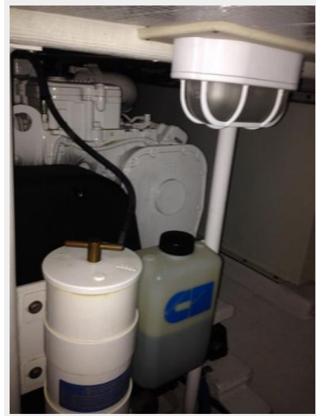
Engine & Mechanical Equipment 5
