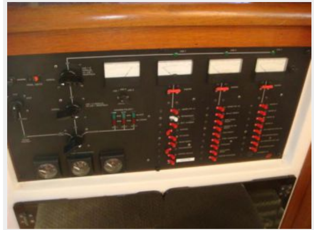
45' Bayliner Electrical Panel
