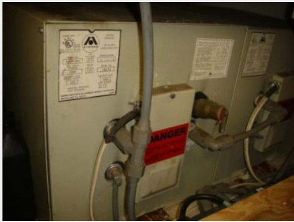
45' Bayliner Water Heater
