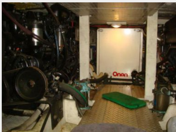
45' Bayliner Engine Room Aft
