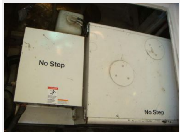
45' Bayliner Generator photo2
