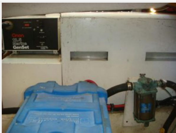
45' Bayliner Generator photo1
