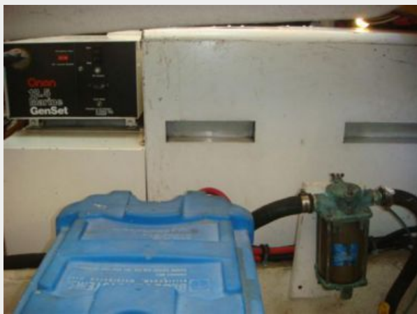
45' Bayliner Generator photo1
