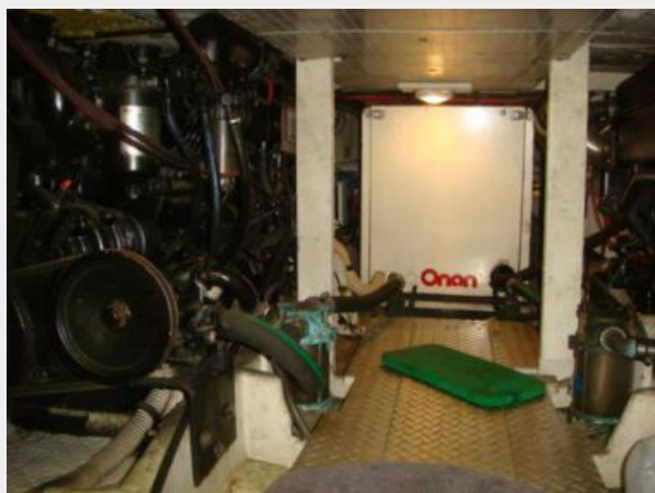
45' Bayliner Engine Room Aft
