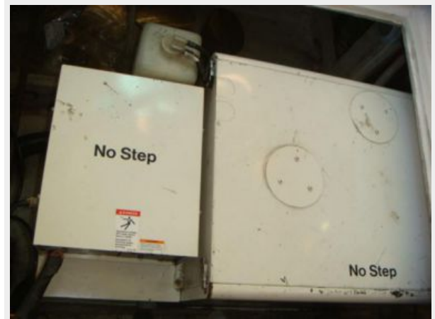
45' Bayliner Generator photo2
