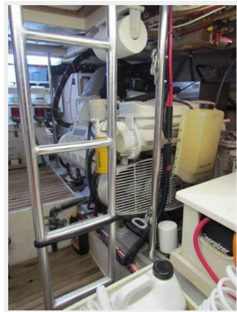
Engine Room Starboard
