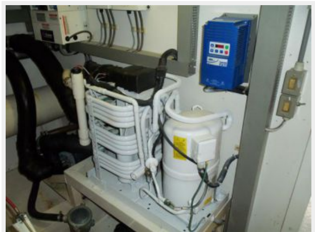
Chilled Water AC
