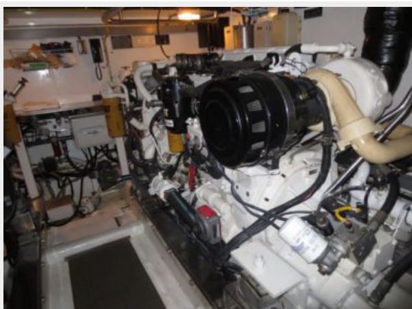
Engine Room C-12 Caterpillar
