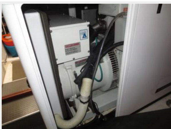
KW Northern Lights Gen Set
