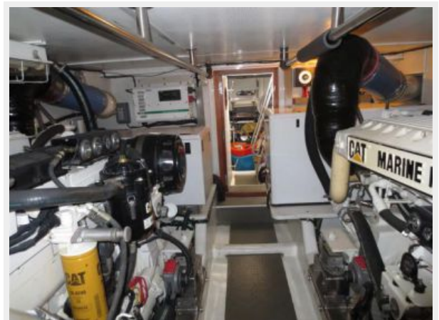
Engine Room Looking Aft
