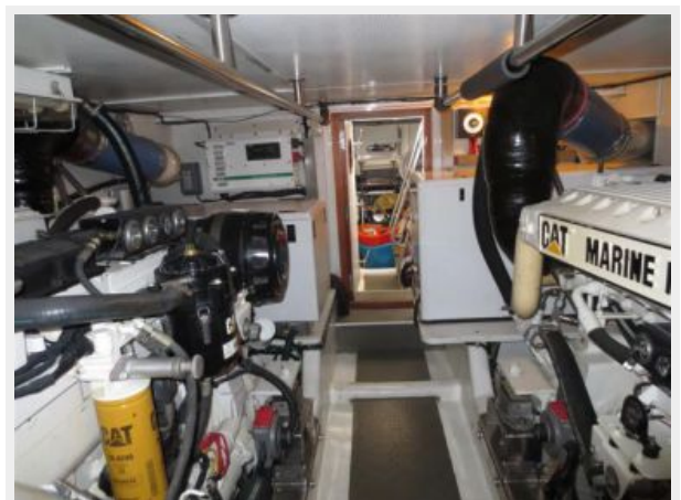
Engine Room Looking Aft
