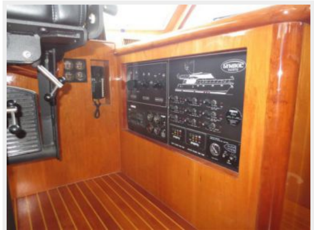
Lower Helm Electronics Panel
