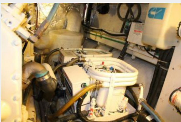
Port Side AC Compressors
