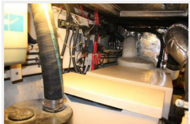
Starboard Side Battery Boxes
