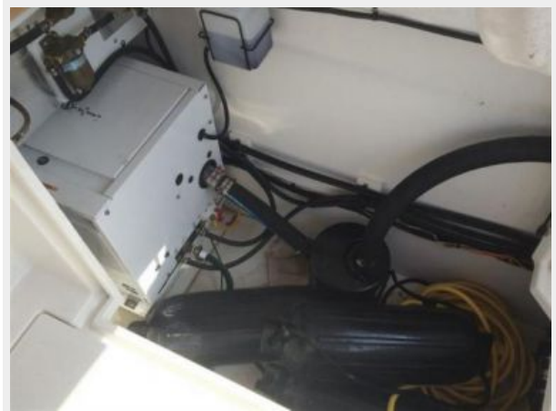
Starboard Engine Area
