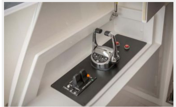
Aft Control Station
