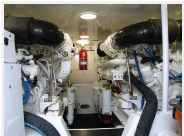
Engine & Mechanical Equipment 1 - Engine Room
