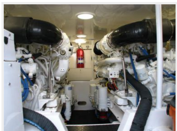
Engine & Mechanical Equipment 1 - Engine Room
