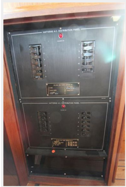
AC distribution panel
