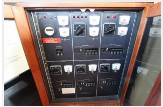
AC electrical panel
