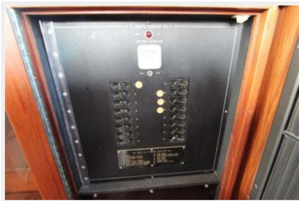
DC electrical panel
