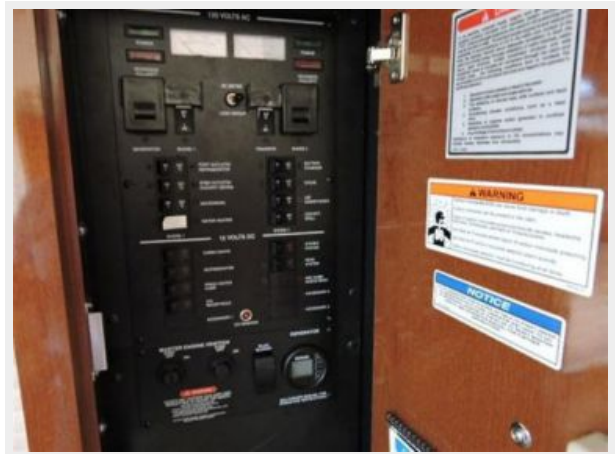
Main Distribution Panel
