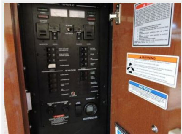
Main Distribution Panel
