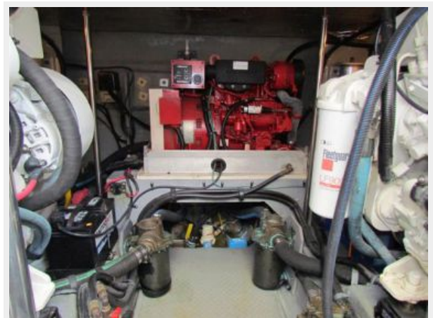
Engine Room Generator
