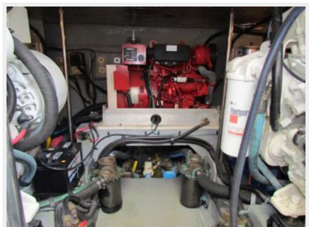
Engine Room Generator
