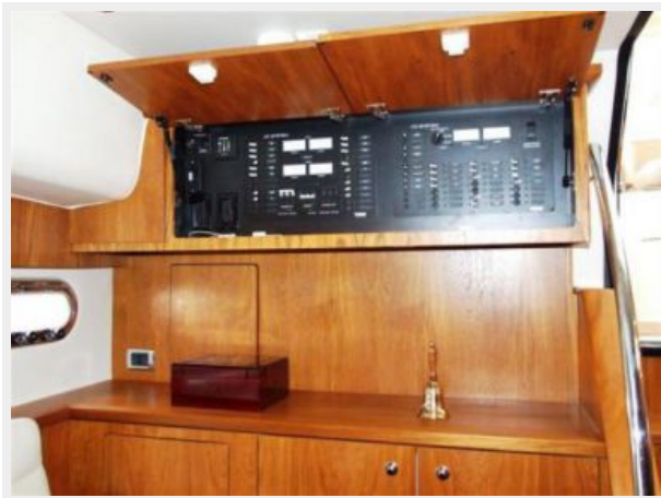
Salon Aft and Electrical Panel
