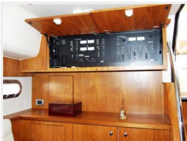
Salon Aft and Electrical Panel
