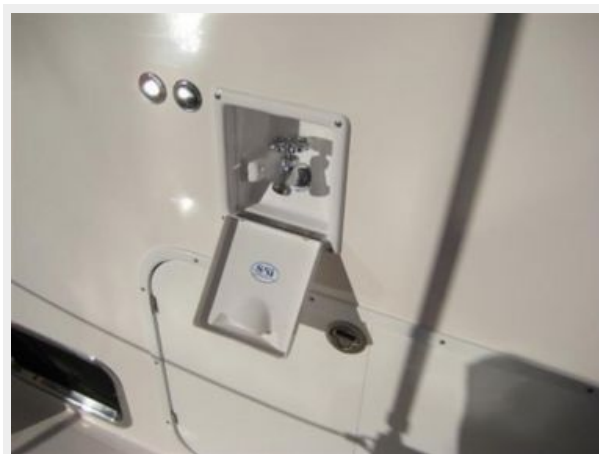
Fresh Water Outlet on Aft Deck
