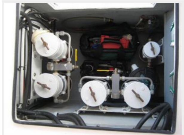
Access to Dual Racors - Engines & Genset
