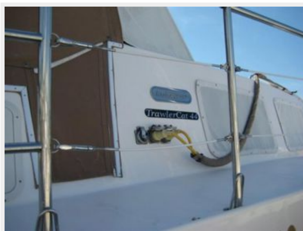
Two 30amp Shore Power Hook-ups
