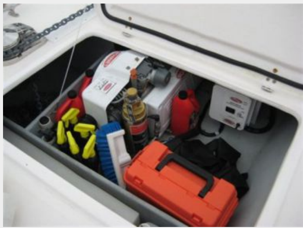
Compressor - Deck Locker, forward starboard side
