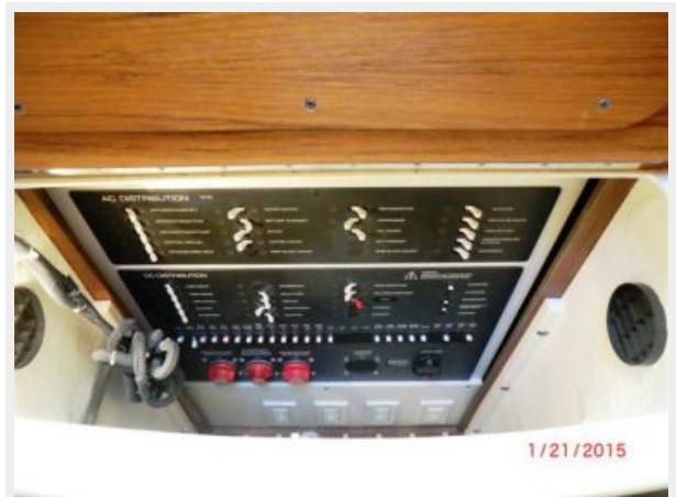
Electrical under Step
