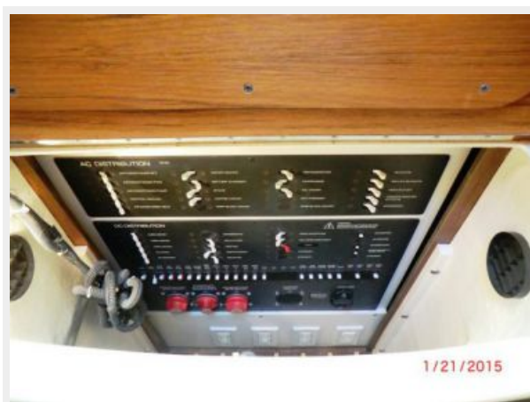
Electrical under Step
