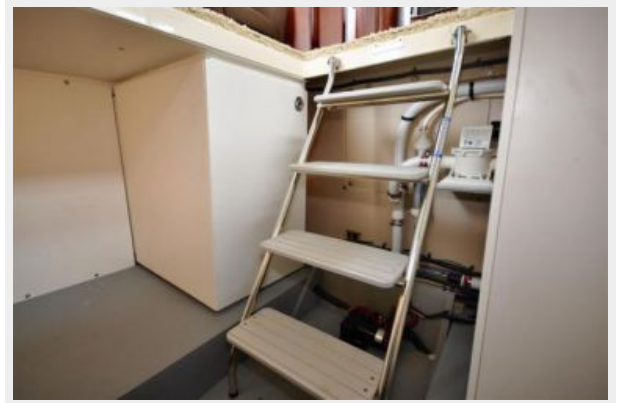
Engine Room Ladder
