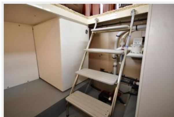
Engine Room Ladder
