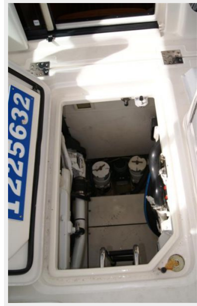
Engine Room Quick Access
