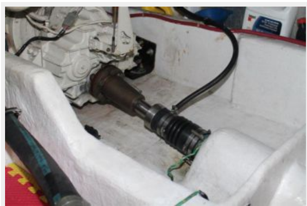
Starboard Shaft and Dripless Seal
