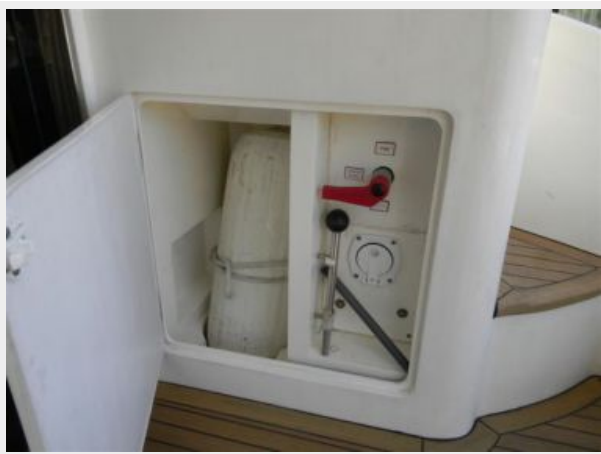
Cockpit Emergency Pump
