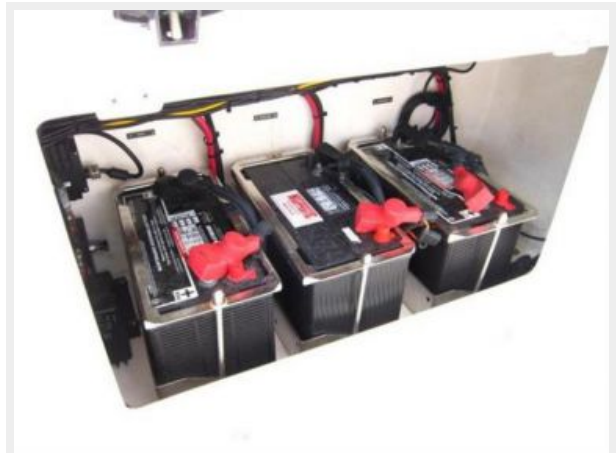
batteries in console
