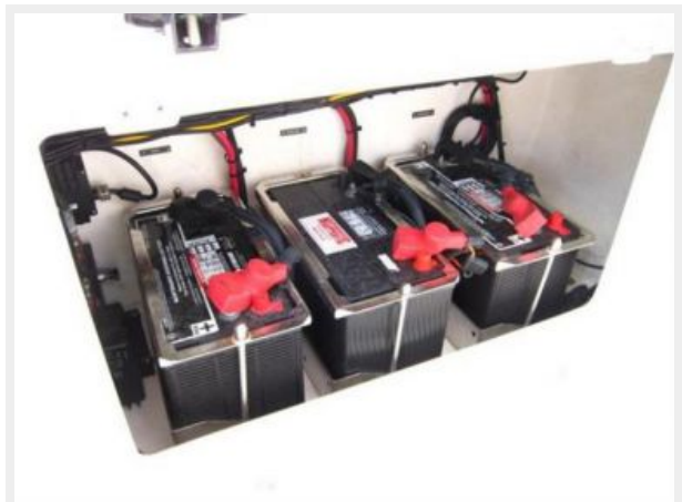
batteries in console
