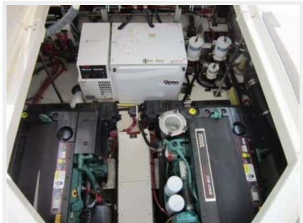
Engine Room Access
