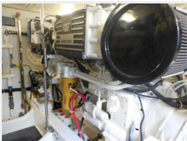
Engine Room - Cat's
