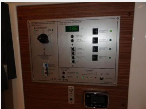
Control Panel (Salon)
