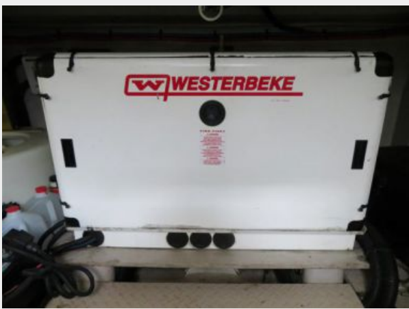
Generator sound shield
