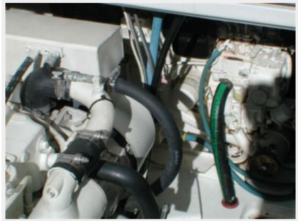
Westerbeke 5KW Generator
