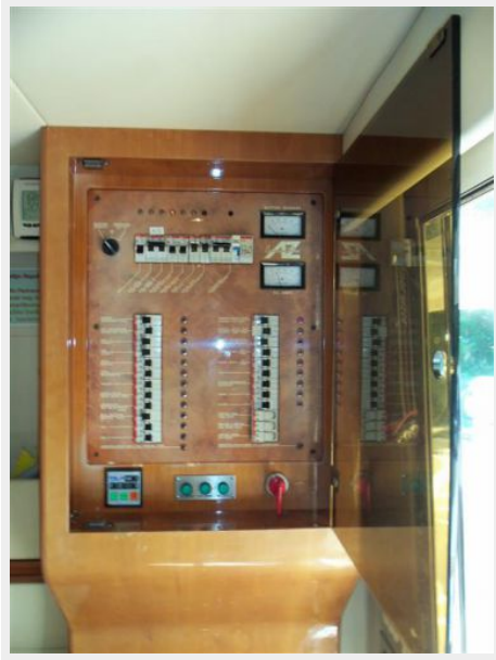
Salon Electrical Panel
