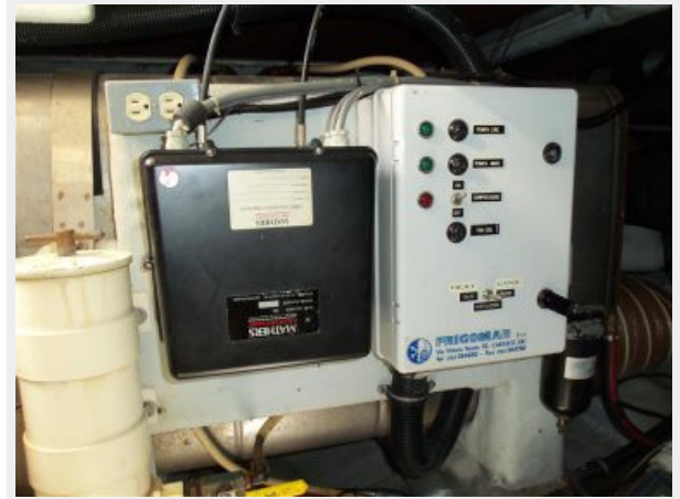
Engine Room Aft to Port
