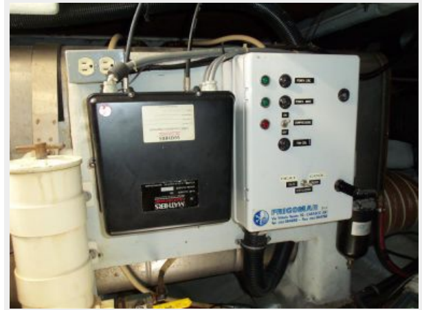
Engine Room Aft to Port
