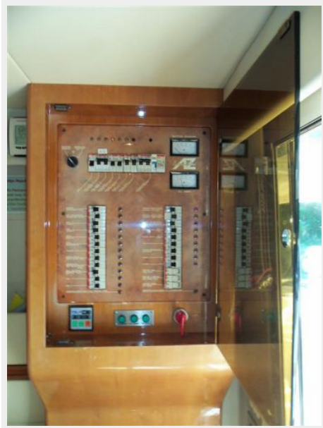
Salon Electrical Panel
