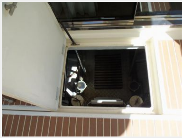
Engine Room Access
