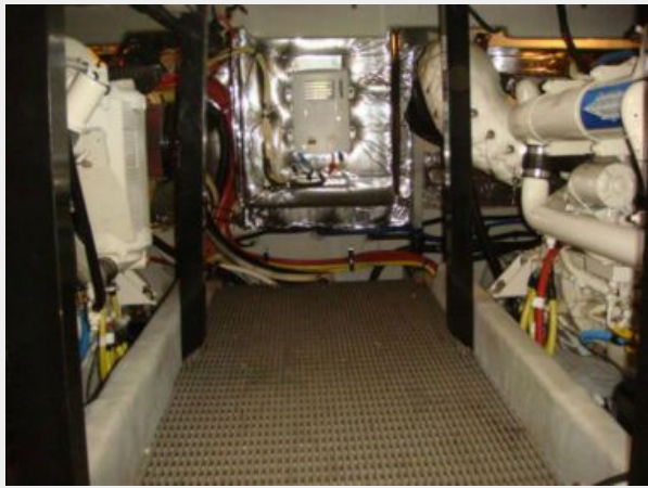
45' Meridian Engine Room Aft
