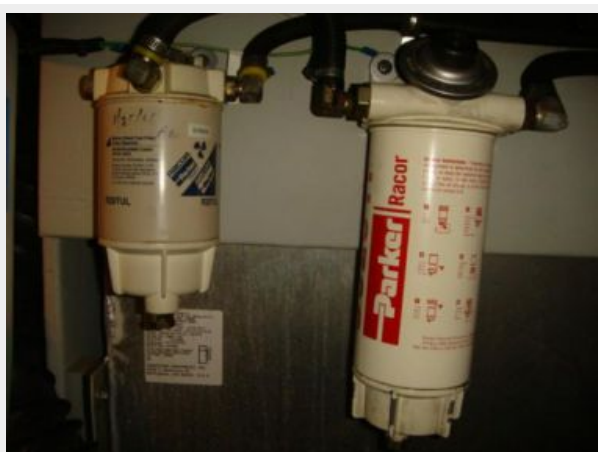
45' Meridian Starboard Racor Fuel Filter
