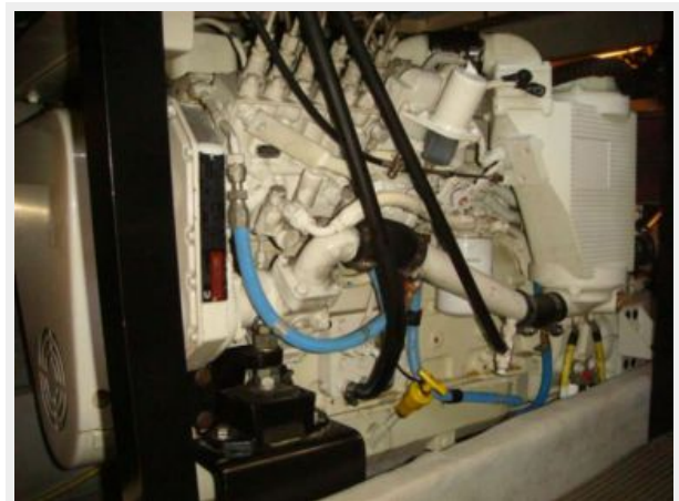
45' Meridian Starboard Main Engine
