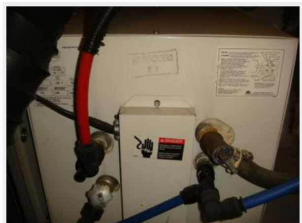
45' Meridian Water Heater
