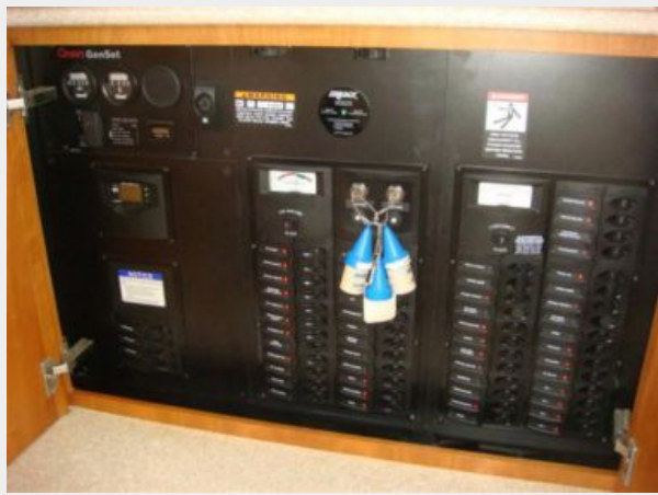
45' Meridian Electrical Panel
