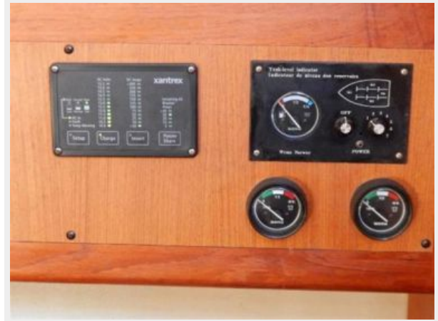
Battery and Tank Monitors
