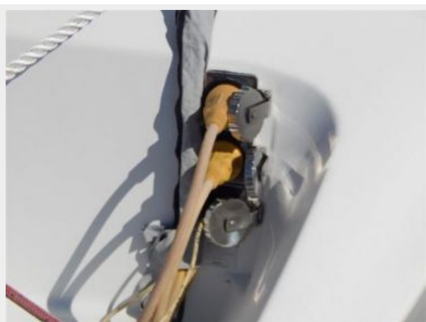
Shore Power Connection
