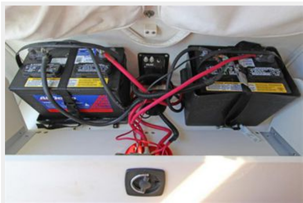
Dual Batteries Mounted In Center Console
