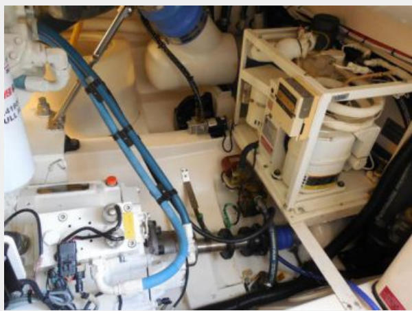
Engine Room Starboard Aft
