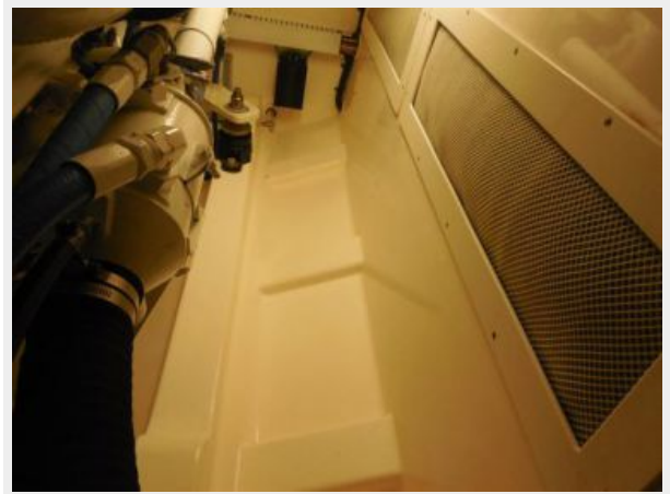
Engine Room Starboard Outboard
