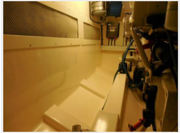
Engine Room Port Outboard
