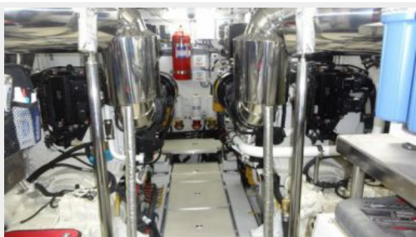
Engine Room Full Beam
