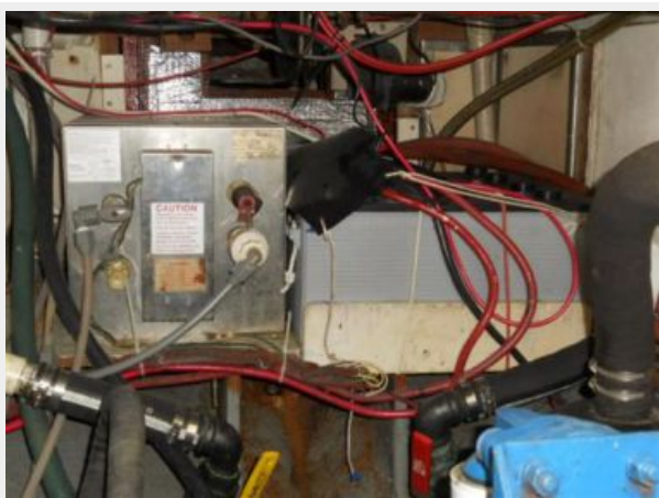
HW Heater / NEW AGM BATTERIES (2014)
