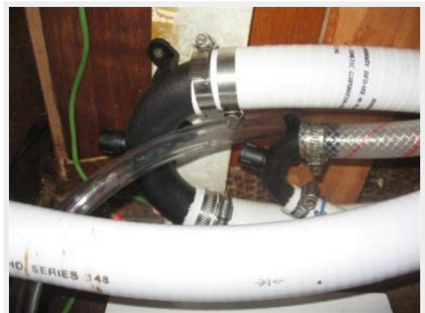
NEW Holding Tank
